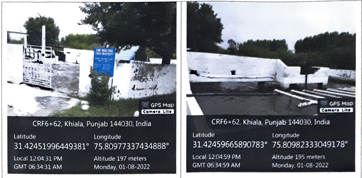
Figure 3. Sewage Treatment Plant
